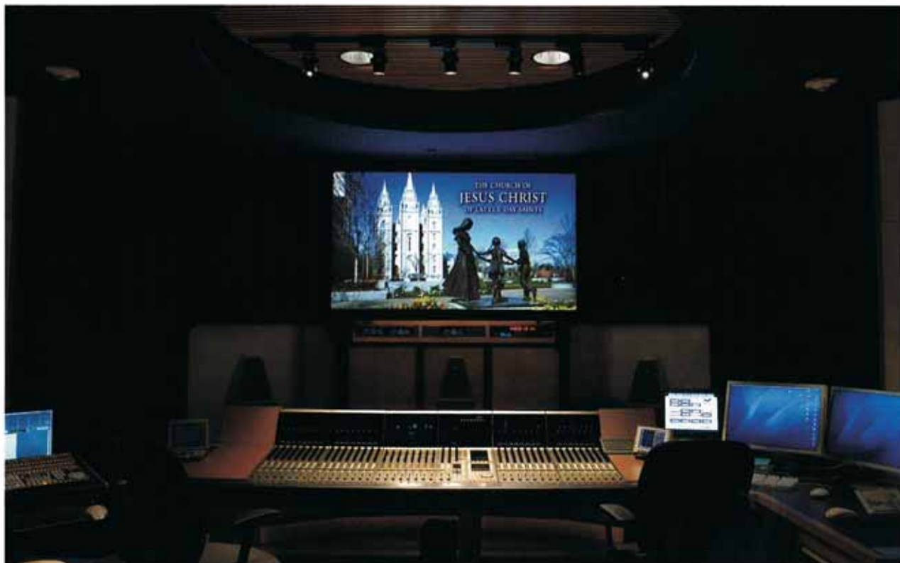
A 32-fader Euphonix System 5-BP mixing console with full redundancy for both power and DSP core is the centerpiece of the multifunctional 5.1 mixing room. It uses the EuCon Hybrid DAW control protocol to enable the surface to control Digidesign Pro Tools HD 7.2, Steinberg Nuendo, and individual DSP channels for editing and post work. A Euphonix R-1 recorder is used as a backup to the Pro Tools mastering system.
